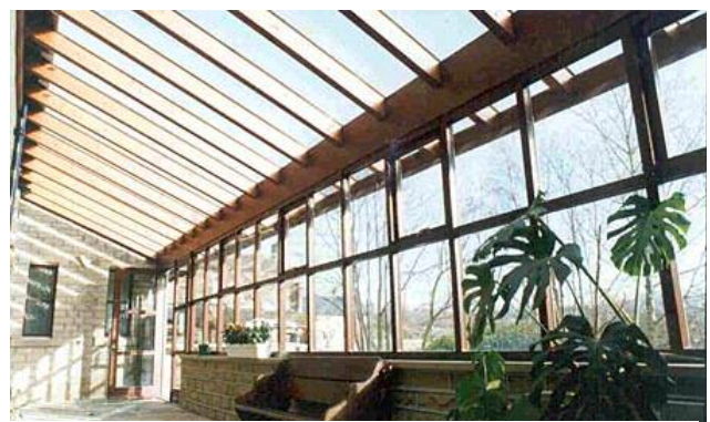
Photo of eco-renovation of Huddersfield Quaker Meeting House on Green Building Store website. ( www.greenbuildingco.co.uk )
